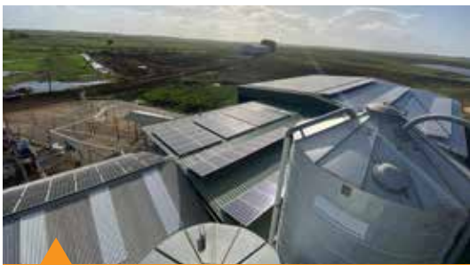
THE INSTALL: 93.3KW ROOF MOUNTED SOLAR SYSTEM
